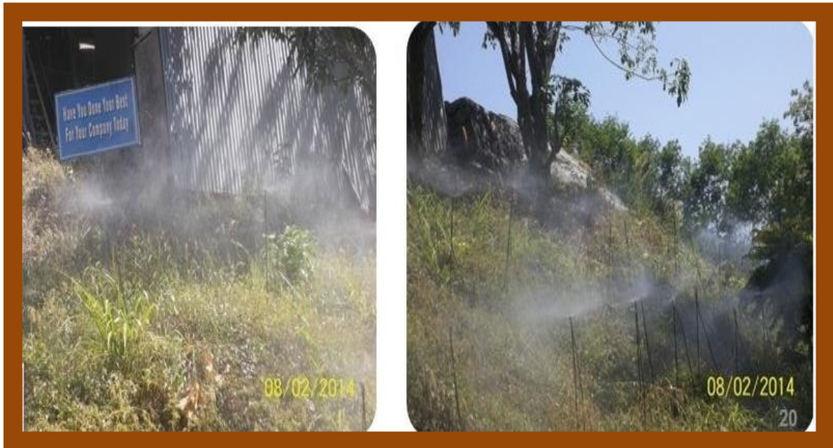
SPRINKLERS INSTALLED AT SITE
